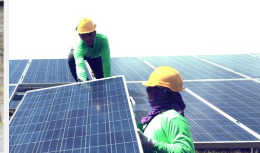
Interport solar system expansion - 250 kWp
