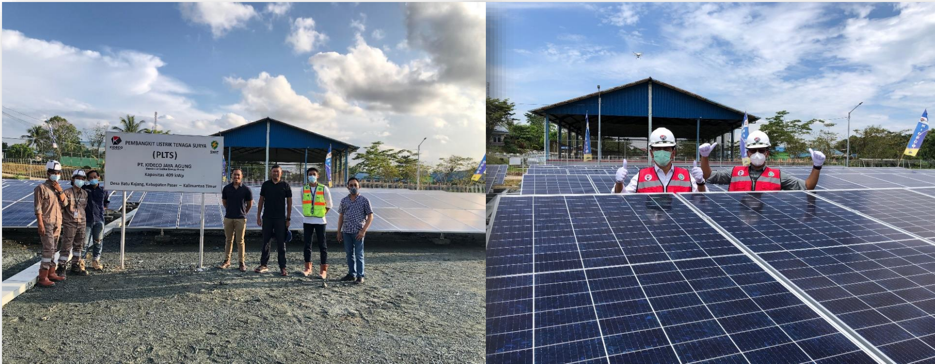
Solar Farm at KIDECO campsite, Batu Kajang Capacity of 409 kWp + Battery 100 kWh
